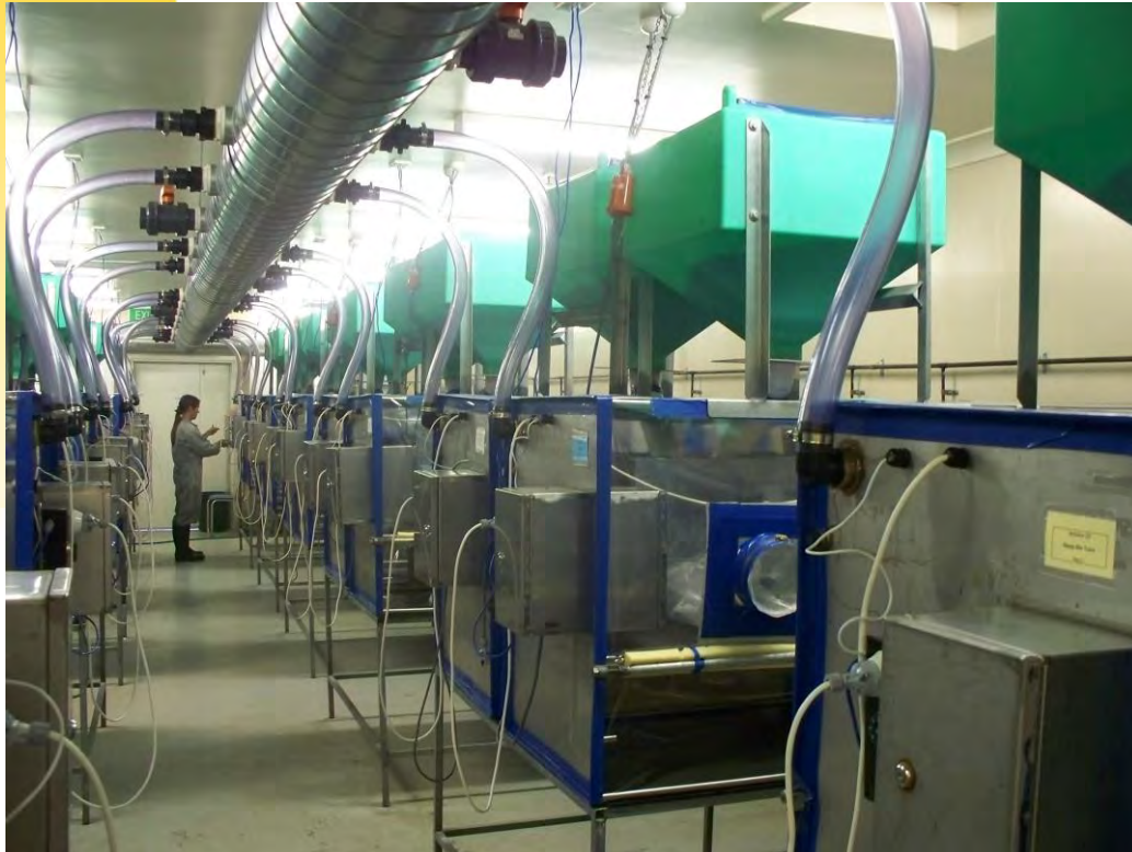
Figure 1-3: Interior of PC2 animal facility containing twenty four (24) isolators, also showing main air inlet duct which carries HEPA filtered, heated air to each isolator
